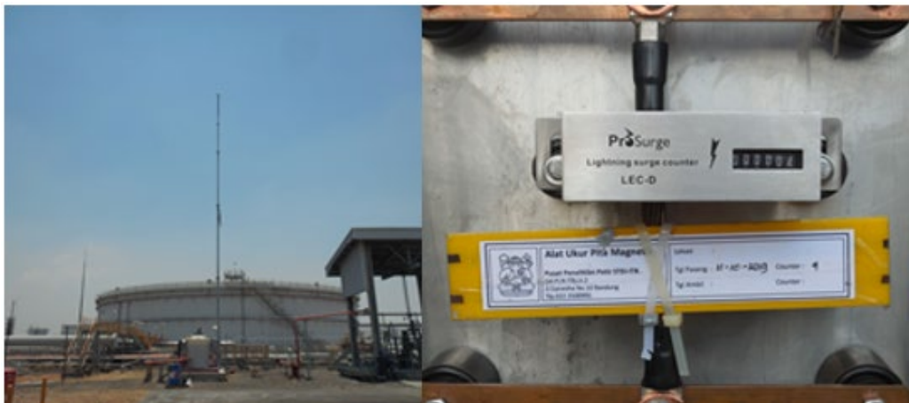
Figure 8. Free standing mast (in Gresik) is equipped by magnetic tape and lightning event counter
